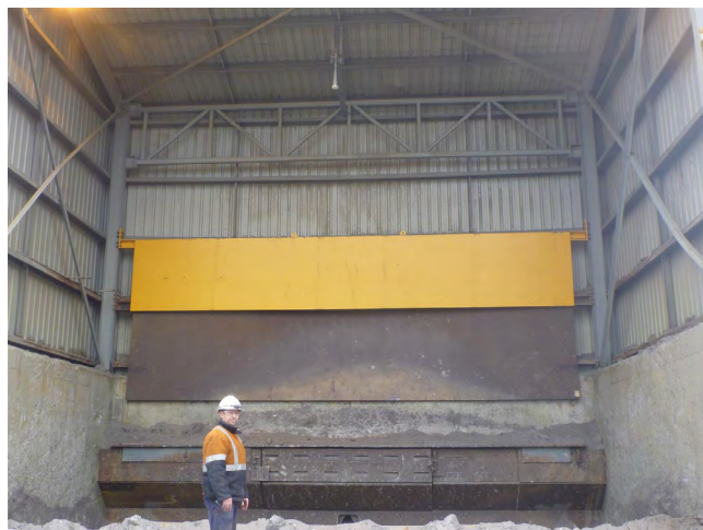
Owen Hocking, Electrical Leading Hand, reviews the installation of the FMR57 in its new position
